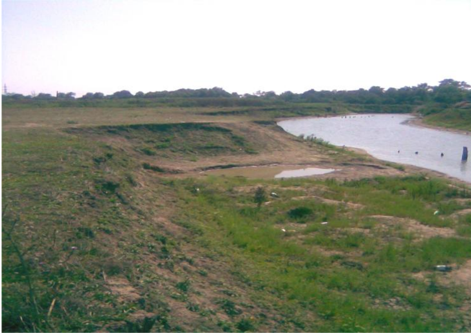
Figure 6: Advanced erosion on the right bank of the meander.
